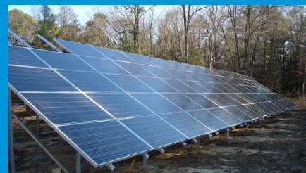
18 kW New Jersey PLM-P235 modules
